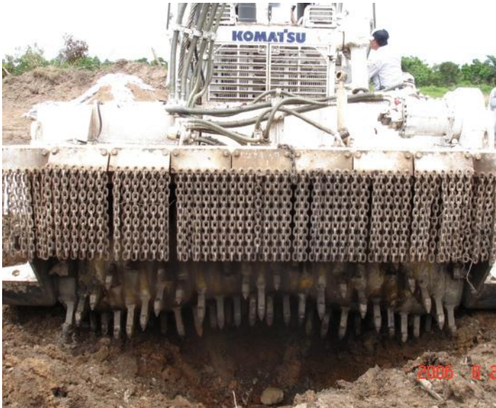
Figure 110: General view of the Komatsu machine after explosion
